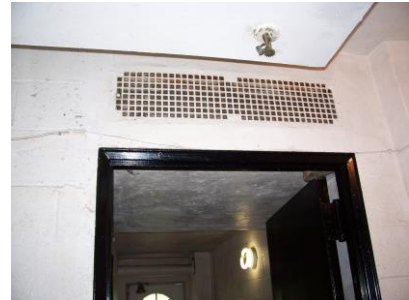
Fig. 27 - Test for adequate air flow in air vents in halls and apartments.
