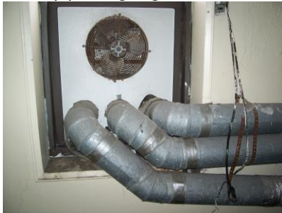
Fig. 28 - Reposition dryer air vents through the wall and seal all penetrations. The above through-the-window method causes heat loss.
