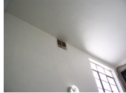
Fig. 33 - Hall light is on when there is sufficient daylight to light the area.
