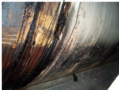
Fig. 8 - Clean and pressure test the tank before introducing No. 2 oil, which acts as a solvent and lead to leaks.
