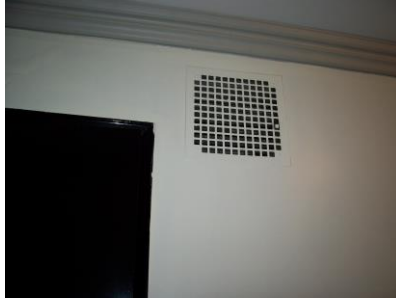
Fig. 23 - Test for adequate air flow in air vents in halls and apartments.
