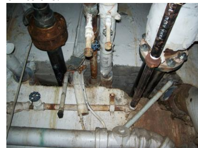
Fig. 9 - Insulating water and steam pipes and sealing holes in walls will reduce heat loss and carbon emissions.
