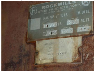
Fig. 2 - The building uses one 1998 Rockmills boiler to heat both buildings.
