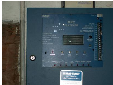
Fig. 5 - Upgrading the Heat Timer system can save energy and reduce carbon emissions by 5 - 15%.
