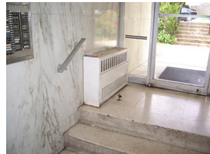
Fig. 18 - Radiator in foyer wastes heat.
