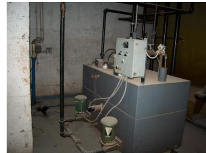
Fig. 6 - Insulating hot water and steam pipes will save energy and reduce carbon emissions.
