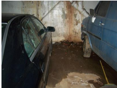
Fig. 26 - Eliminate water leaks in garage.
