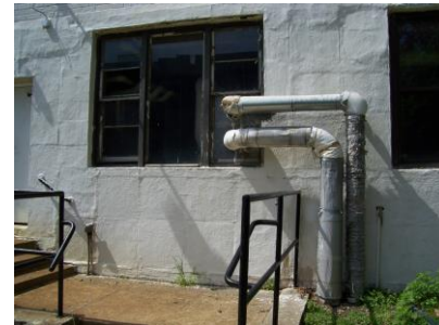
Fig. 3 - Connecting the boiler to the other building through a window may not comply with NYC DOB Code.
