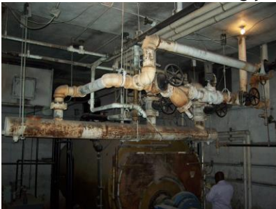
Fig. 1 - The boiler room will be brought up to current Code requirements, including insulating all pipes greater than 3" in diameter.
