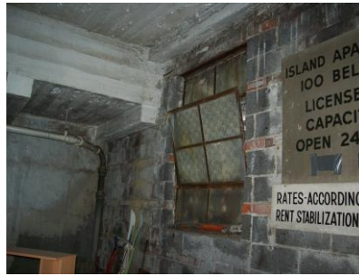
Fig. 14 - Replace garage window to reduce heat loss from DHW pipes overhead.
